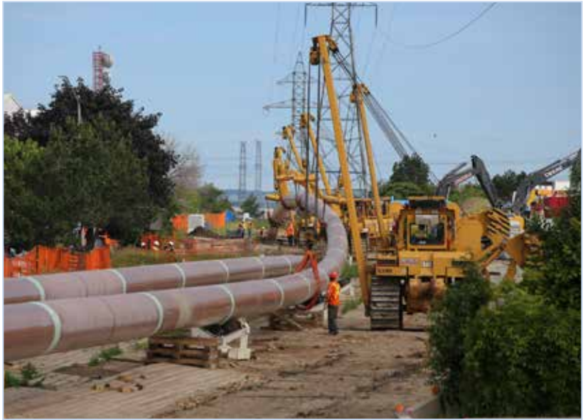
Michels Canada Co. constructing Enbridge Gas Distribution Inc.'s largest project in history
